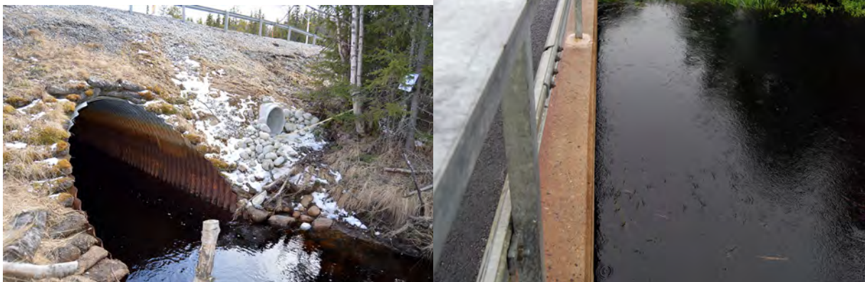
Picture 8. Dry culvert next to a wide culvert (ID 97, Långbäcken). The dry culvert has been used very much by different species of animals.
