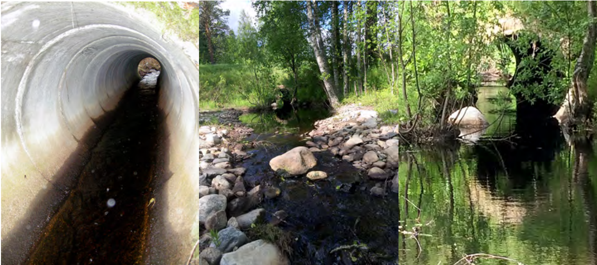
Picture 4. The picture to the left shows a culvert with high and low water depth. The pictures in the middle and to the right show the site following the construction of a rocky ridge downstream the culvert. Due to the rocky ridge, the water level has increased and the water velocity is reduced (ID 280).
