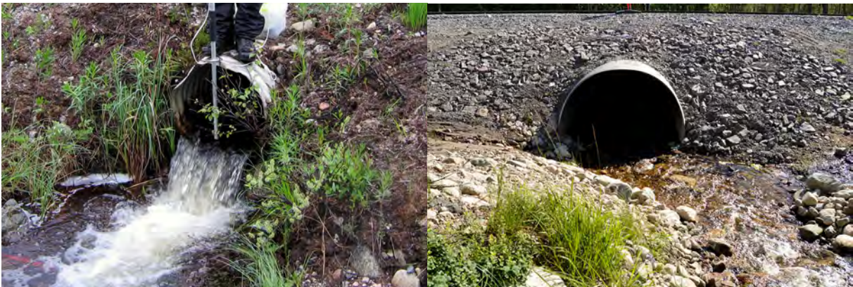
Picture 3. The picture to the right is showing a culvert with high water velocity and with a drop at the outlet. The picture to the right is showing the same site after the culvert has been replaced with a wider culvert and a recreated stream bed (ID 54).
