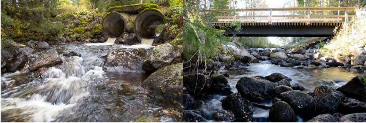
Picture 2. The picture to the left is showing a double culvert with high water velocity and with a drop at the outlet. The picture to the right shows the same site after the culverts have been replaced with a bridge (ID244).
